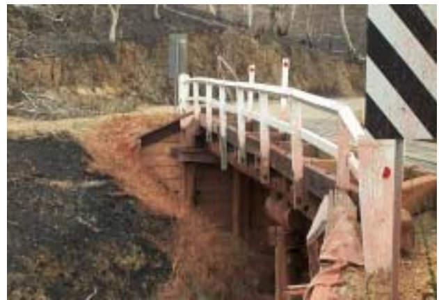
Bingo Munjie Creek Bridge - showing traces of the "Phos-Chek" fire retardant
